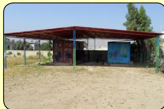
The new metal- and woodworkshop.
